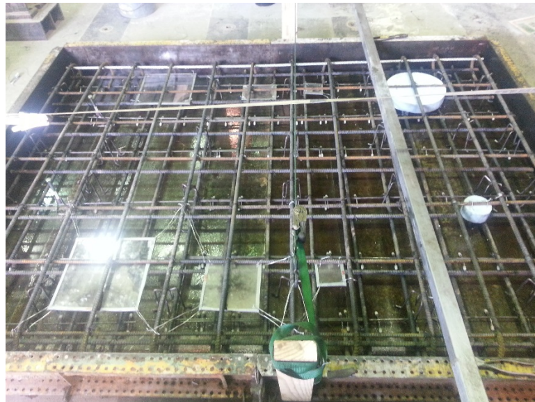
Figure 5.7. Photo of formwork and rebar cage for mock-up bridge deck containing artificial defects before casting.
